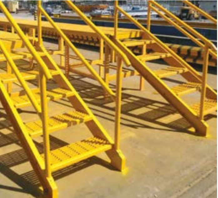
Serrated Stair Treads in Operation Platform
